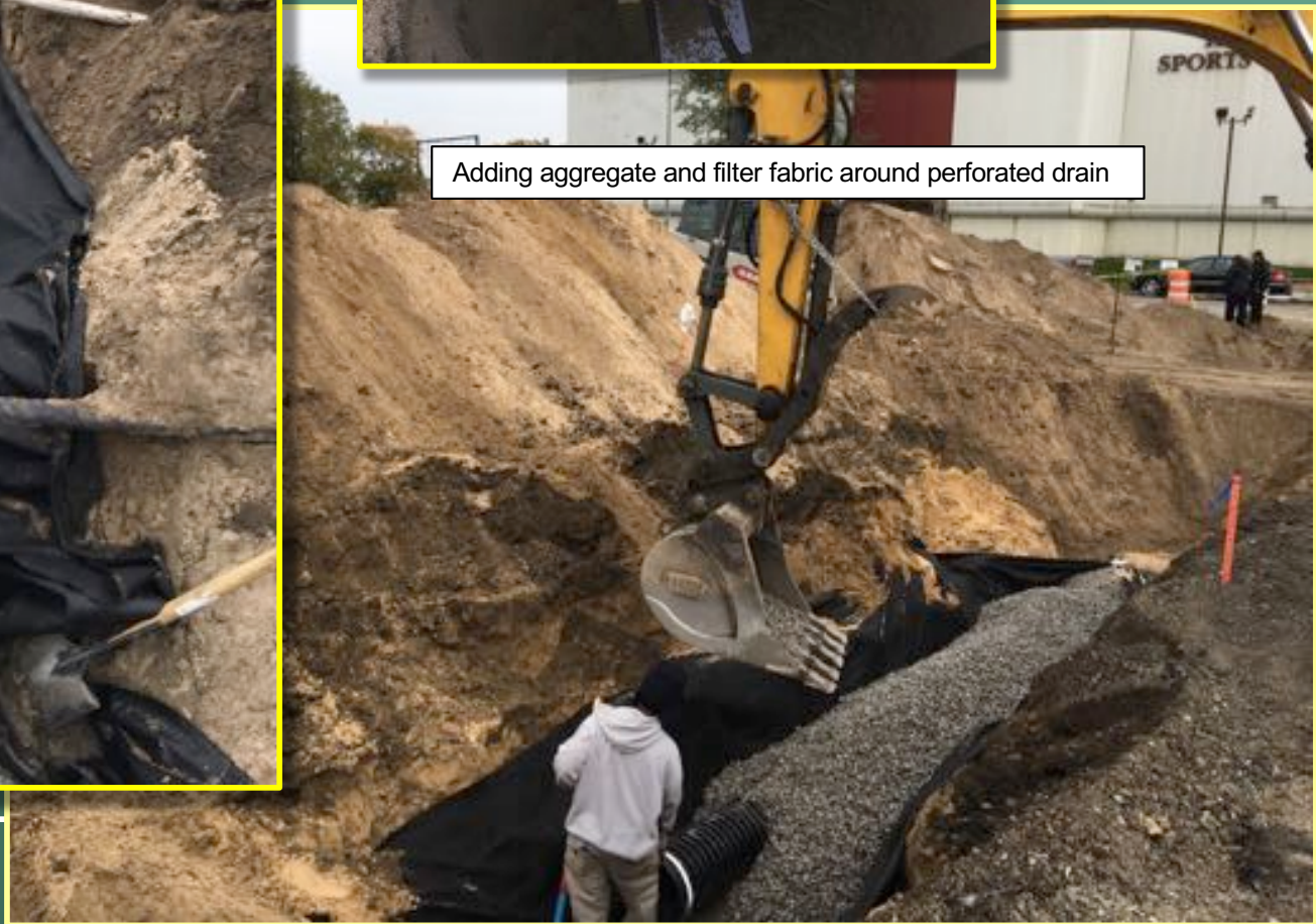
Soil moisture sensors were installed above and below the perforated drain in order to measure infiltration.
